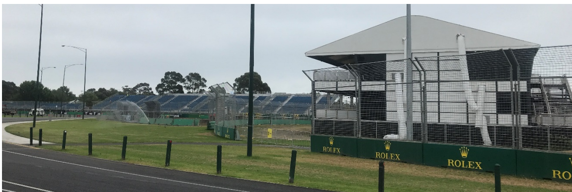
Construction of the circuit for the April 7-10 event started in January and is well advanced. The photo (taken 28/2/22) shows the 'Chicane' corporate pavilion facing Turn 1 and a row of huge grandstands .
